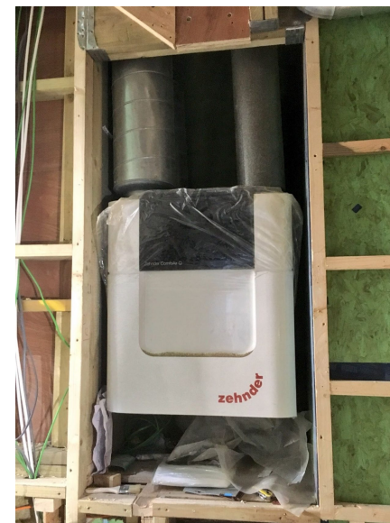
Image of Zehnder MVHR unit being retrofitted into an existing house (Source: Bow Tie Construction)
